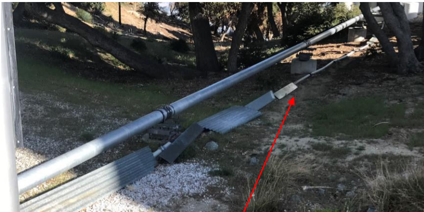
Current fiber conduit for ALOHA Runs along ground
